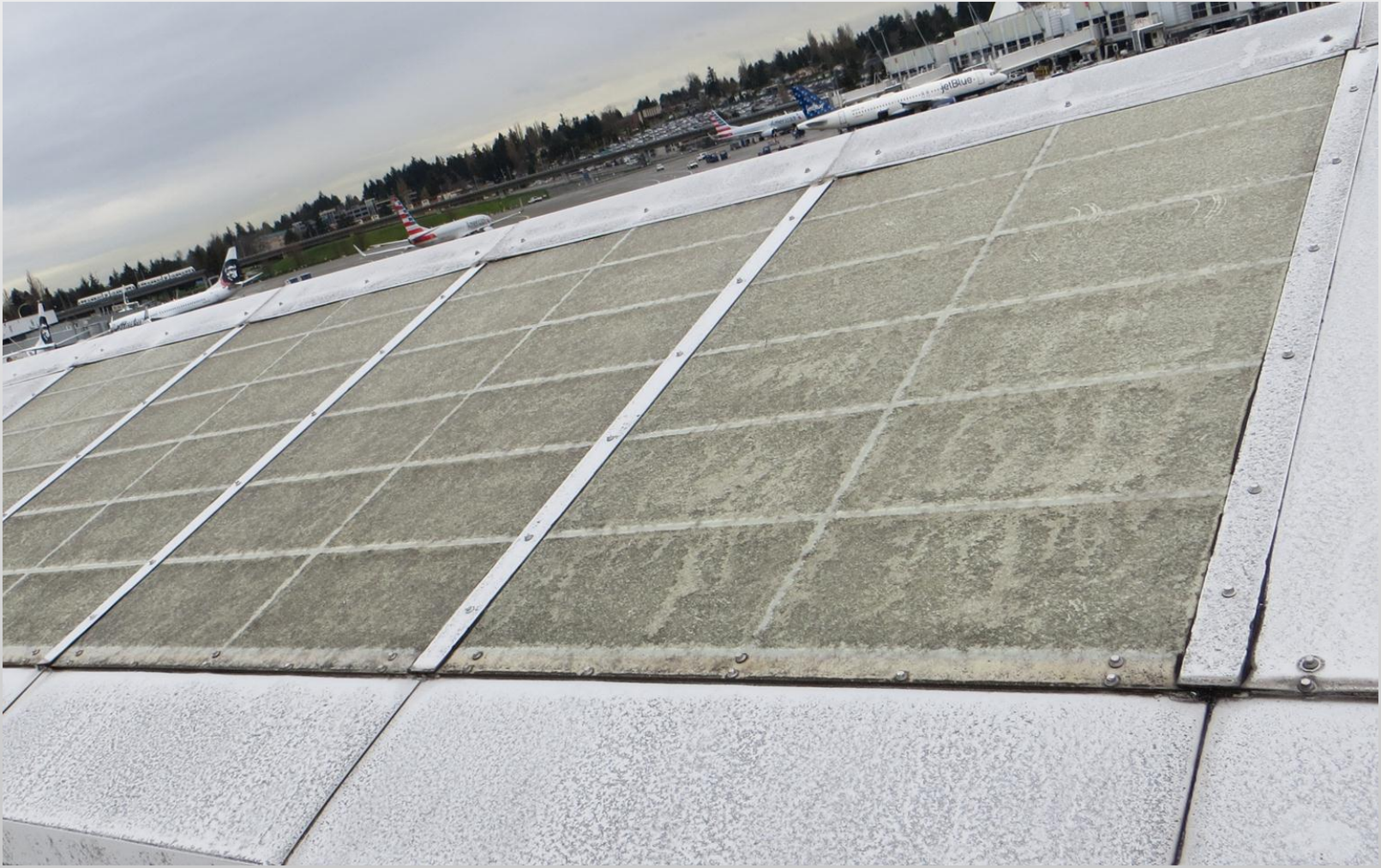
Kalwall skylight panels – beyond their useful life expectancy
